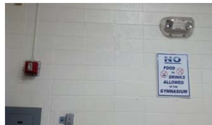
Typ. Emergency Lighting Fixture
