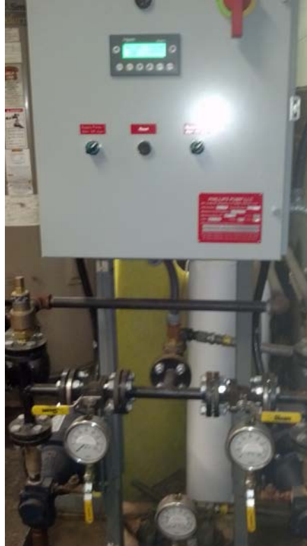
Fuel Oil Pumps
