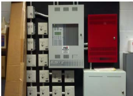
Fire Alarm Control Panel
