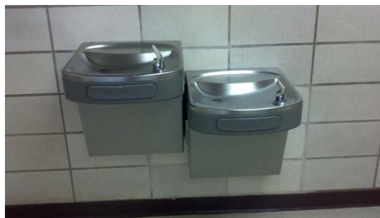
Existing Electric Water Coolers
