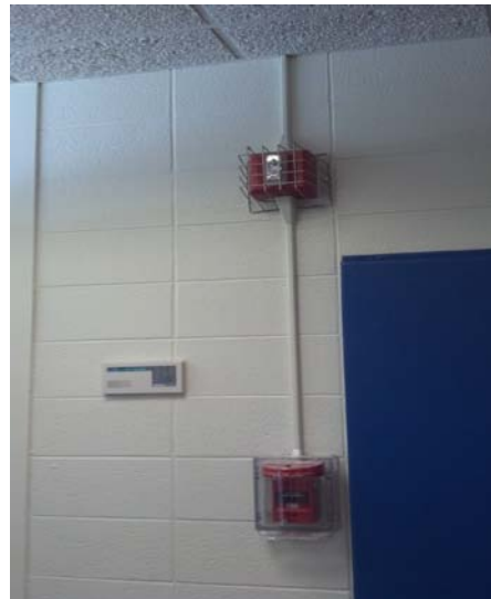
Typical Fire Alarm Pull Station and Audio-Visual Device
