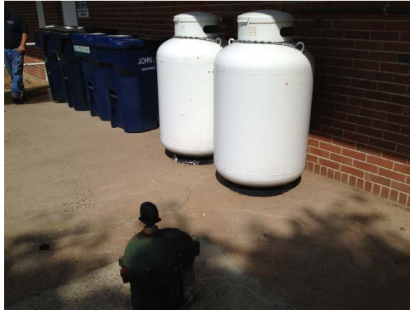
Existing propane tanks
