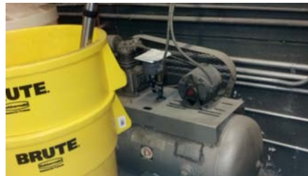
Control System Compressor
