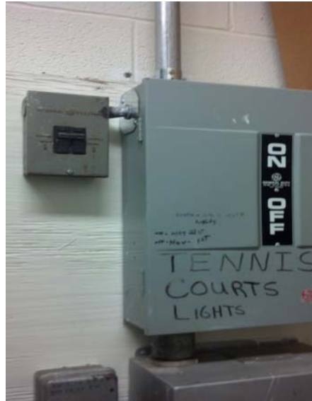
Tennis Court Disconnect Switch
