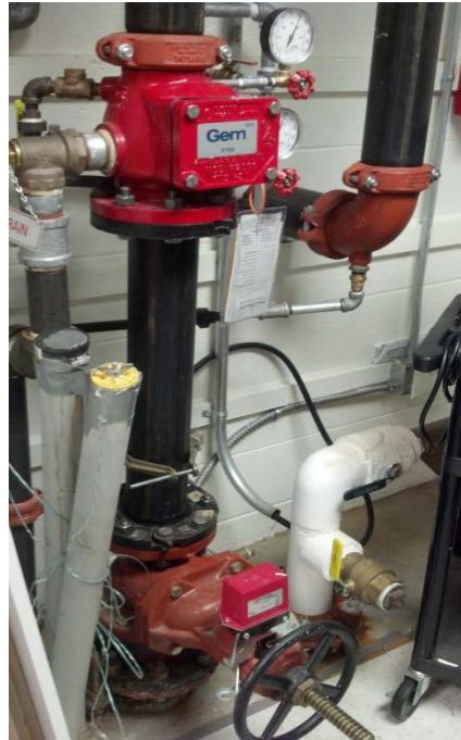
Existing Fire Service Riser
