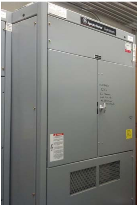
Main Electrical Switchgear
