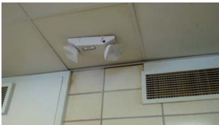
Typ. Emergency Lighting Fixture
