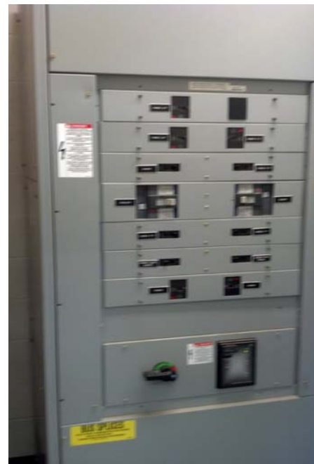
Main Electrical Switchgear
